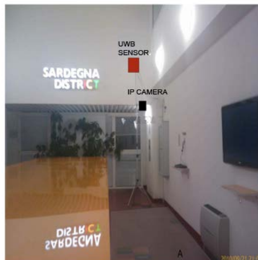
Figure 23 Area of system installation. Focus on the "A" area.
